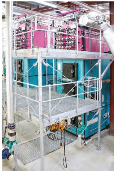
The Biomass boiler at Zealandia Horticulture in Canterbury.
