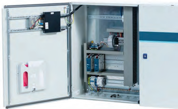
Priva controllers, an easy user-interface showing all data at the growers fingertips.
